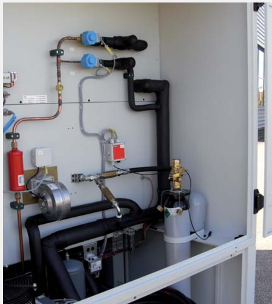
Flame extinguishing system
